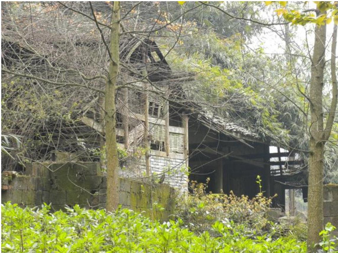
Figure A.3.84. Earthquake Damage to a Chaping Resident of a Rural Community
