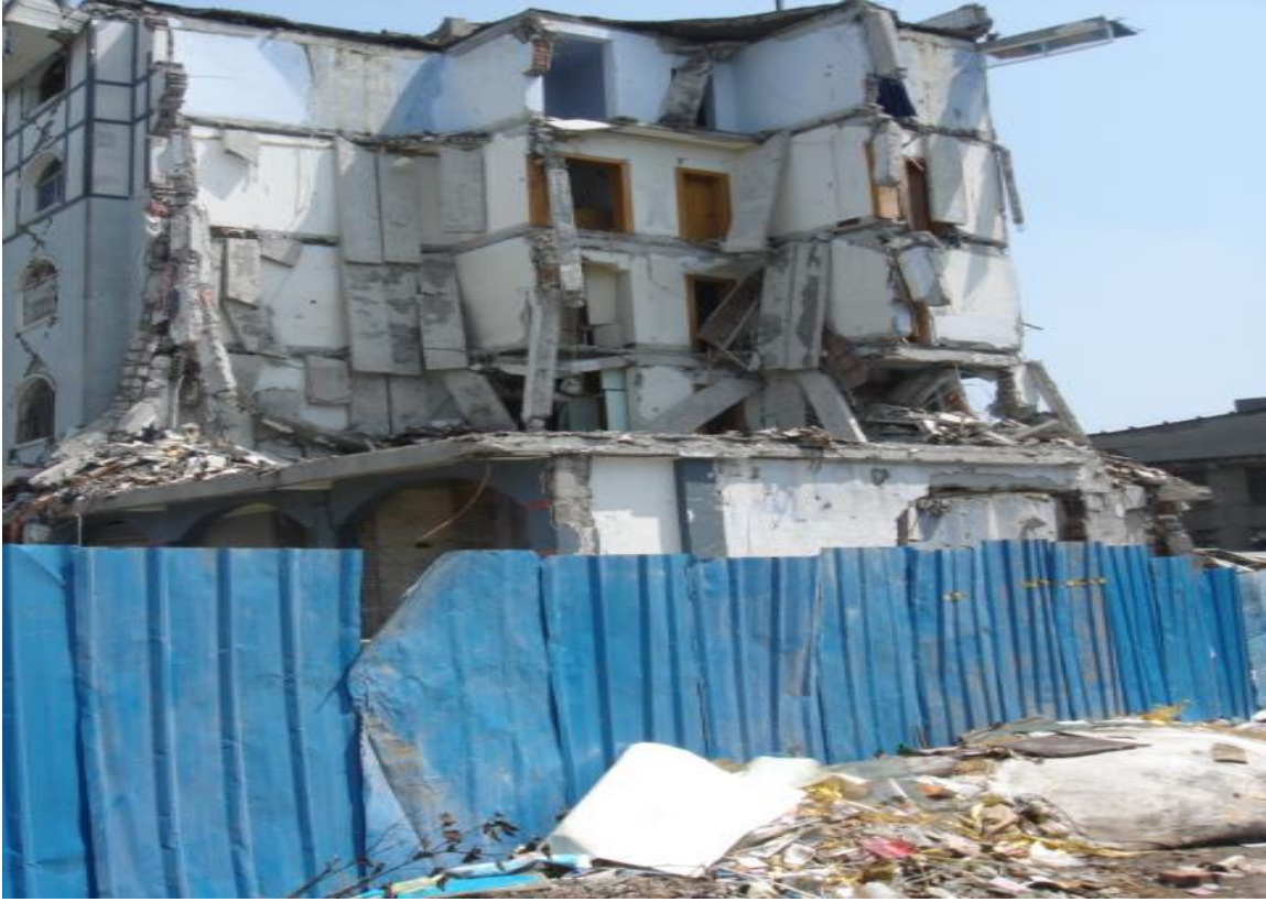
Figure 1.2. Destruction of a Residential Building in Dujiangyan (Source: Photo taken by Jia Lu, 2008)
