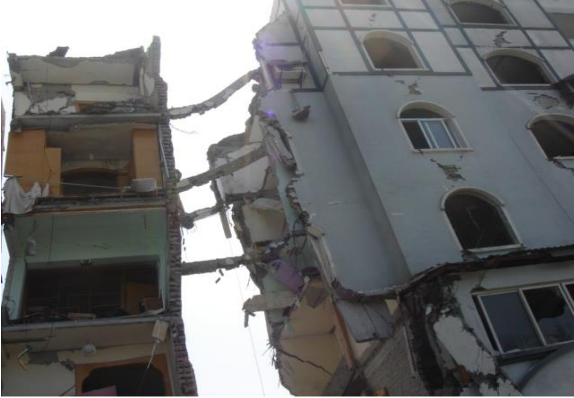
Figure 1.1. Near-collapsed Buildings in Dujiangyan (Source: Photo taken by Jia Lu, 2008)
